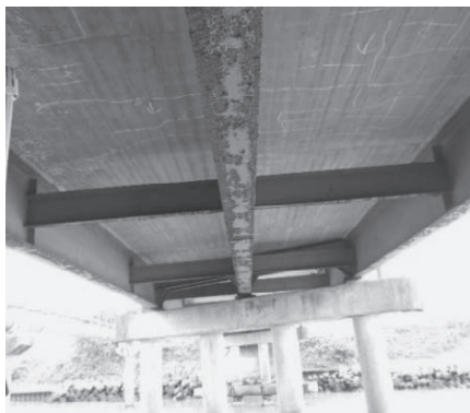
(c)上部構造の腐食
